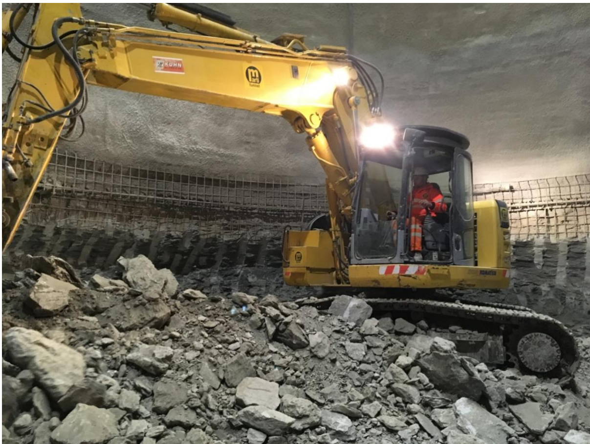
Figure 1: Excavation of a shaft for the PM17 shaft at CERN in molasse ground (OPEN-PHO-ACCEL-2018-008, Copyright by CERN).
